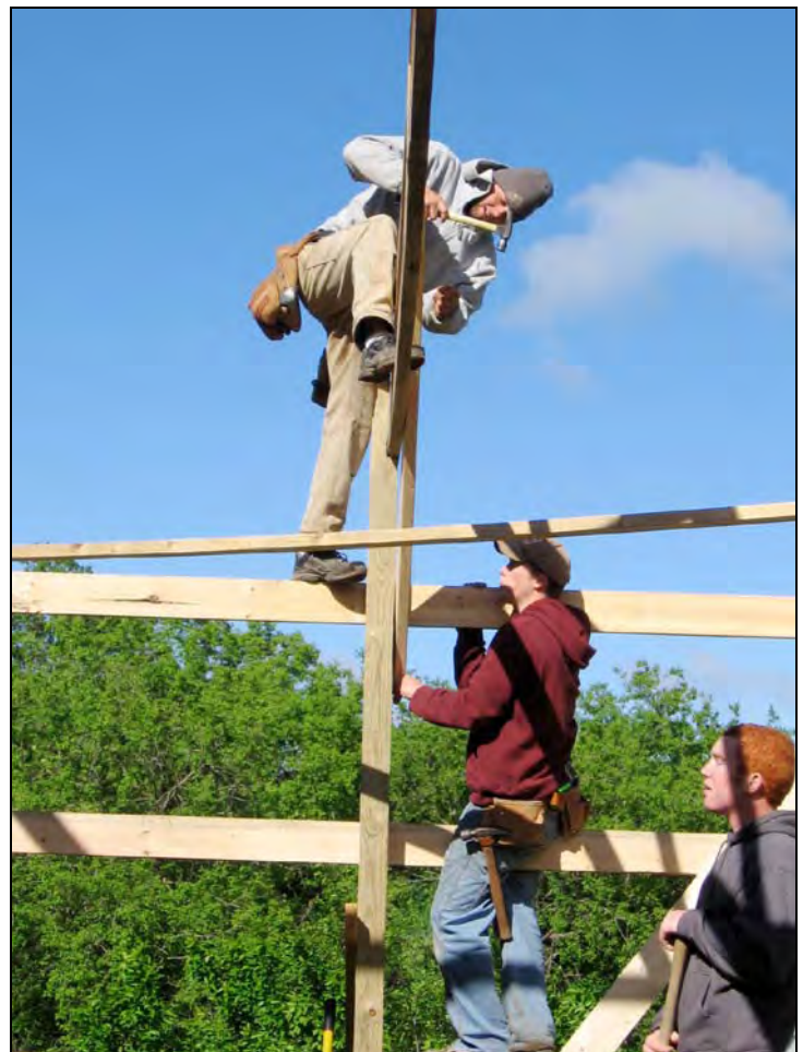
Josiah Hylden, Jesse Kallender, and Tim Ostberg are helping to secure the trusses of the new storage shed.
