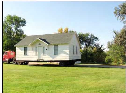
The Zion cabin was moved from its previous location of northeast of the chapel, onto a new foundation just south of Bethel. This was to facilitate the chapel move. The new foundation for this cabin was also accomplished with the help of the summer staff and volunteers.
