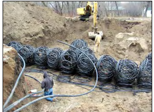
The field for geothermal heating and cooling.
